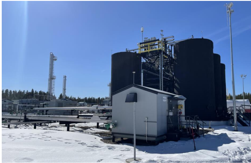
Figure 6: Atmospheric tanks at gas plant
