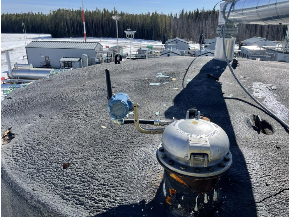
Figure 8: Wireless open/closed position monitoring of thief hatch
