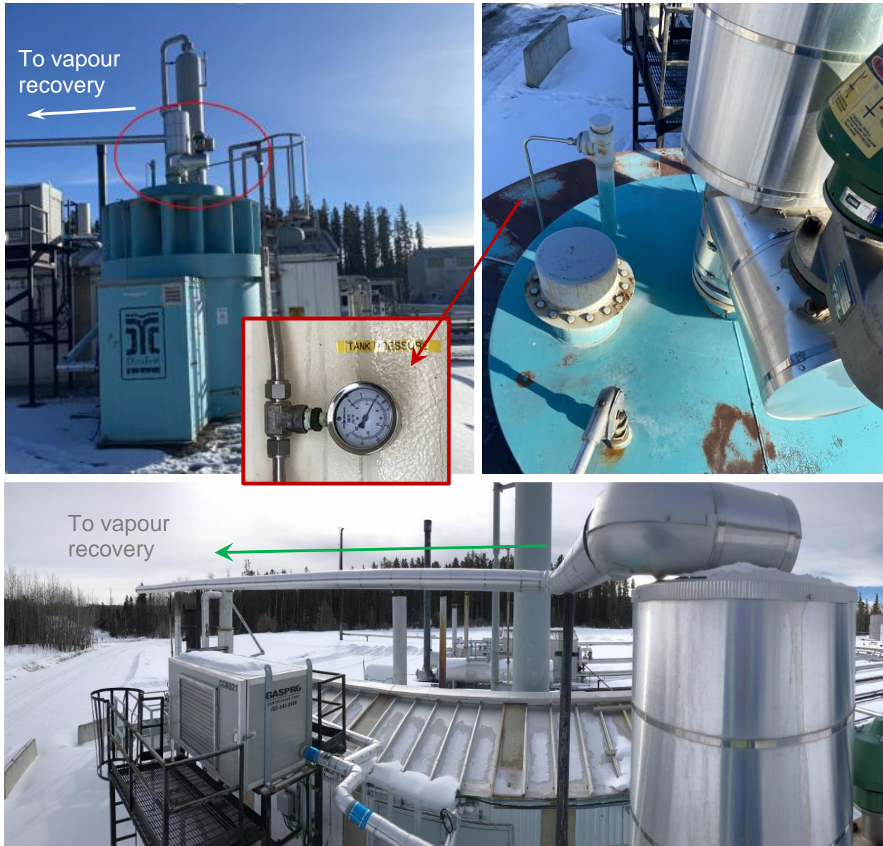
Figure 15: Production tank with vapour recovery and sensing line for pressure indication
