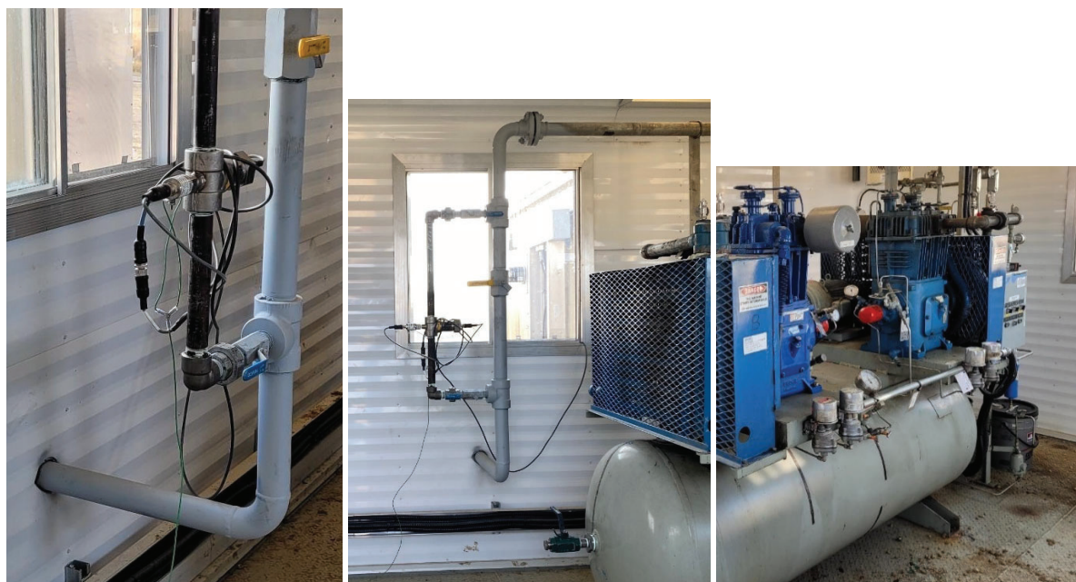
Figure 3: Ventsentinel® meter installed on discharge from air compressor with remote monitoring
