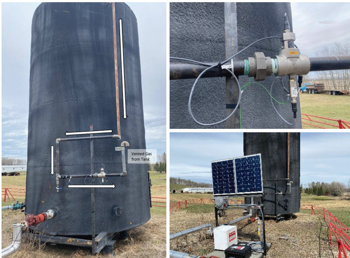
Figure 2: Ventsentinel® meter installed on 400-bbl tank with remote monitoring infrastructure to remotely data log the ongoing flow measurements and other measurement variables
