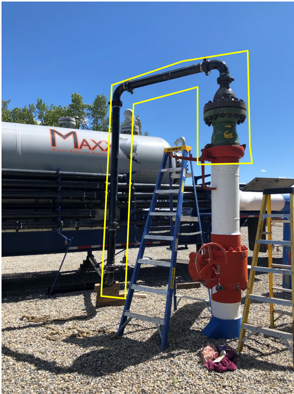
Figure 9: During equipment set-up of Pilot #2. The NPS 12 blowdown riser on the right served as the connection point for the temporary piping to the P-tank and then incinerators.
