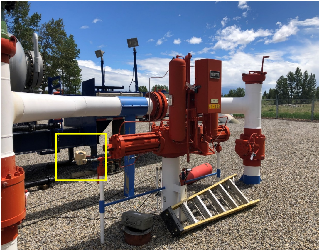
Figure 10: Pressure gauge located upstream of the separator tank which allowed for monitoring of the pipeline pressure during the incineration event.
