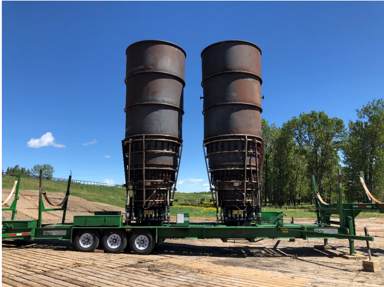
Figure 6: TCI Incinerators being set up on site. Matting had been installed several days prior.
