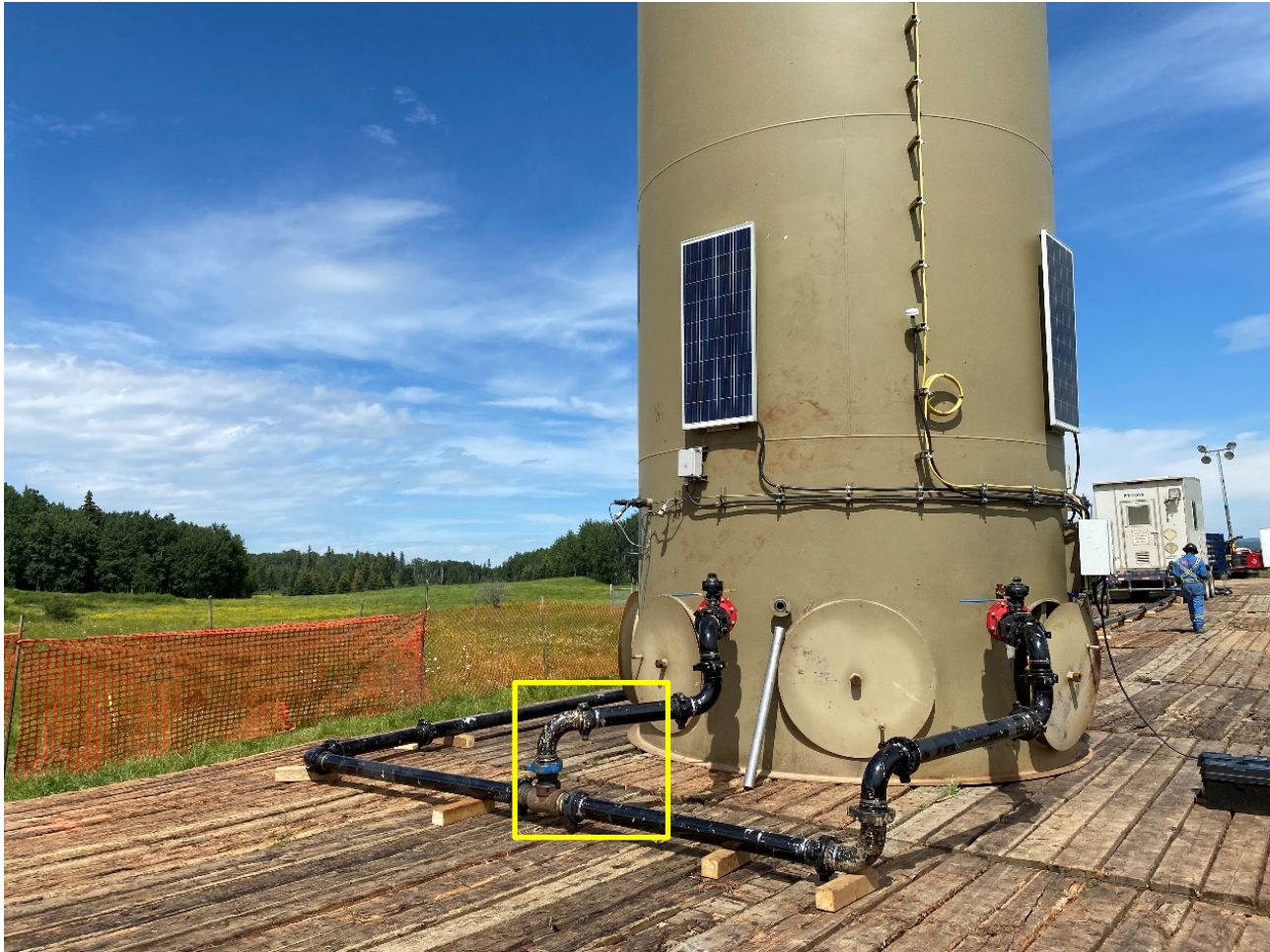
Figure 14: NPS 4 and NPS 6 NPT tapped flange connection. Ties from temporary piping to connect to each incinerator unit.
