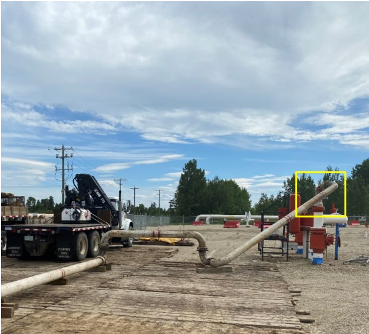
Figure 13: During equipment set-up of Pilot #3 with temporary piping connecting from the P-tank (not in the picture – starting on the far left) to the pipeline riser (on the right).
