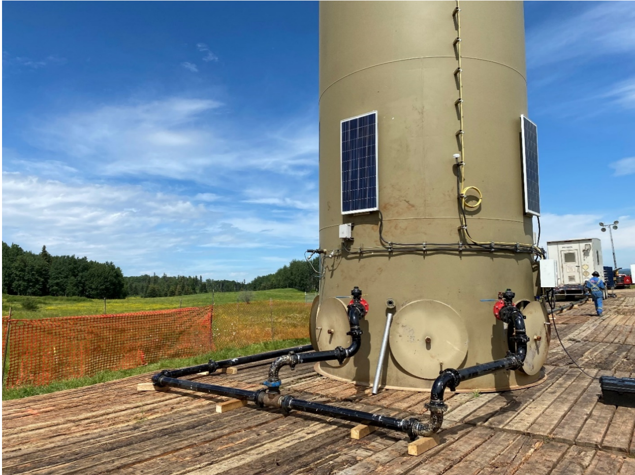
Figure 7: Questor incinerator being set-up on site. Matting had been installed the day prior to equipment set-up.
