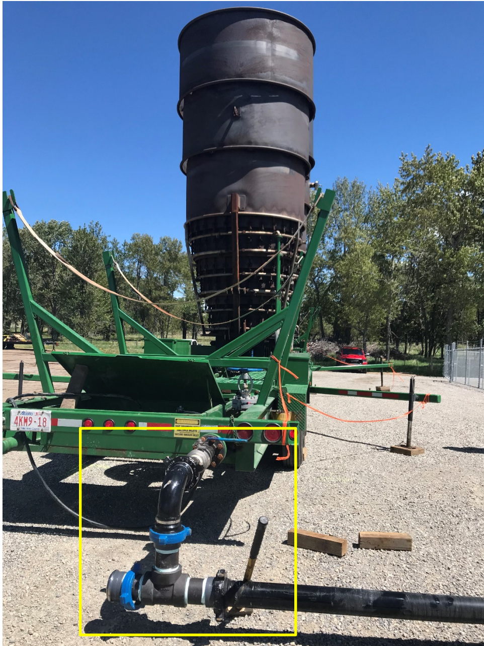
Figure 11: NPS 3 NPT tapped flange connection. Tees from temporary piping to connect to each incinerator unit.
