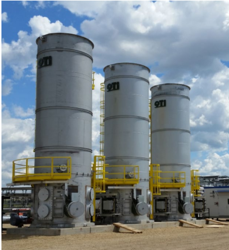
Figure 2: Questor Technology Inc. Q-5000 Permanent Incinerator Units at a Rail Car Loading Facility in Edmonton
