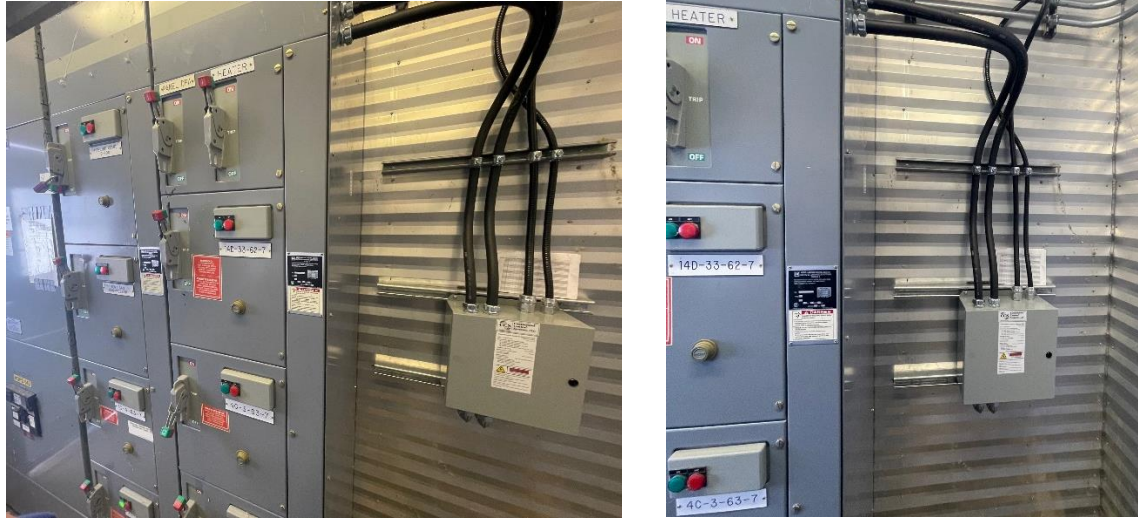
Figure 4 – MCM in the Small Building
