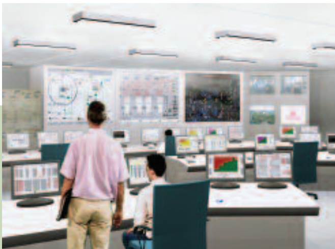
The ergonomics of the EPR control room benefits from the latest developments (computer-generated picture).
