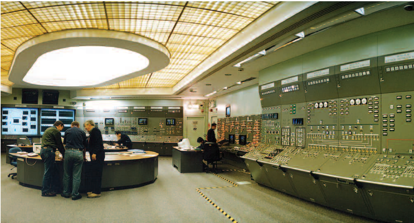
Figure 2-21 Main Control Room (Qinshan)
