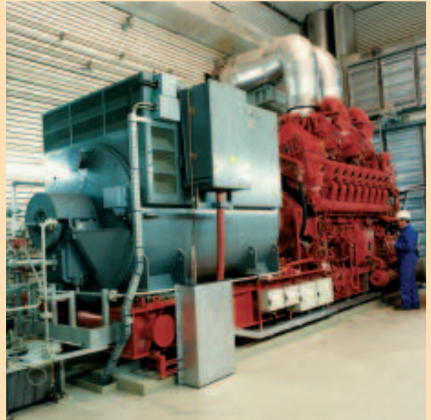
Isar 2, Germany (Konvoi, 1,300 MWe) emergency Diesel generator.
