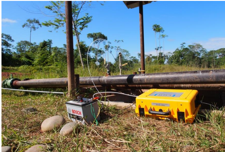
Figure B.6: Downstream sampling of the acetylene in the flare line at Auca Sur 1 using a multi-hole sampling probe connected to the CRD gas analyzer.
