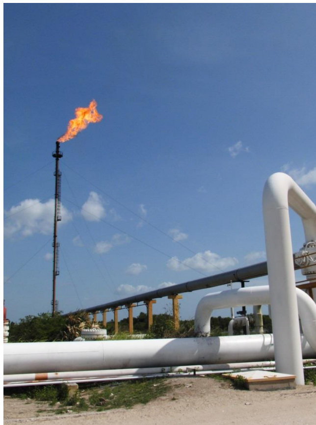
Figure A.2: Southern emergency flare at the Atasta compressor station in Campeche, Mexico.
