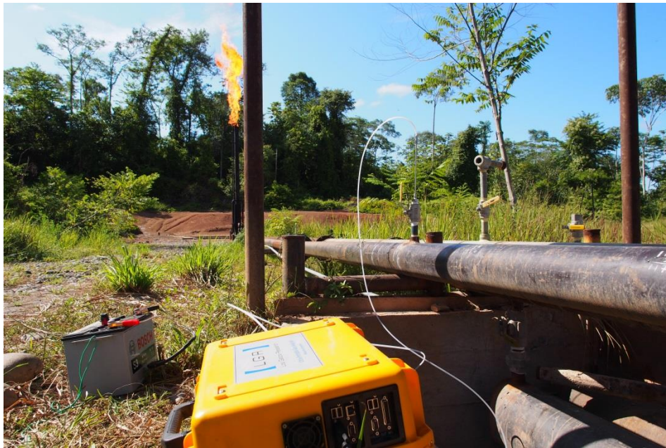
Figure C.6: Flare at Auca Sur 1. Pictured are three hot taps on three adjacent lines, each line had an additional hot tap upstream (not shown). The centre line of the three terminated at a blind flange just after the hot tap pictured. The other two lines were the subject of flow rate measurements.
