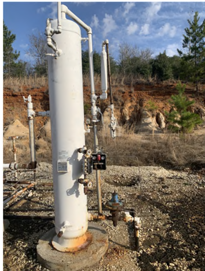
Figure 1. Photo of the Well Test Site Separator
