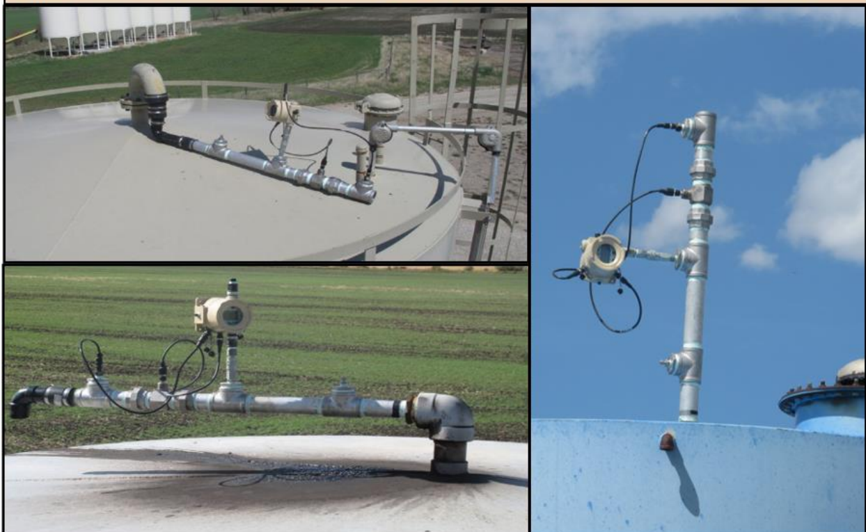
Figure B-12: Calscan's Hawk 9000 Data Logger with 2" Gas Turbine and T&P Sensors
