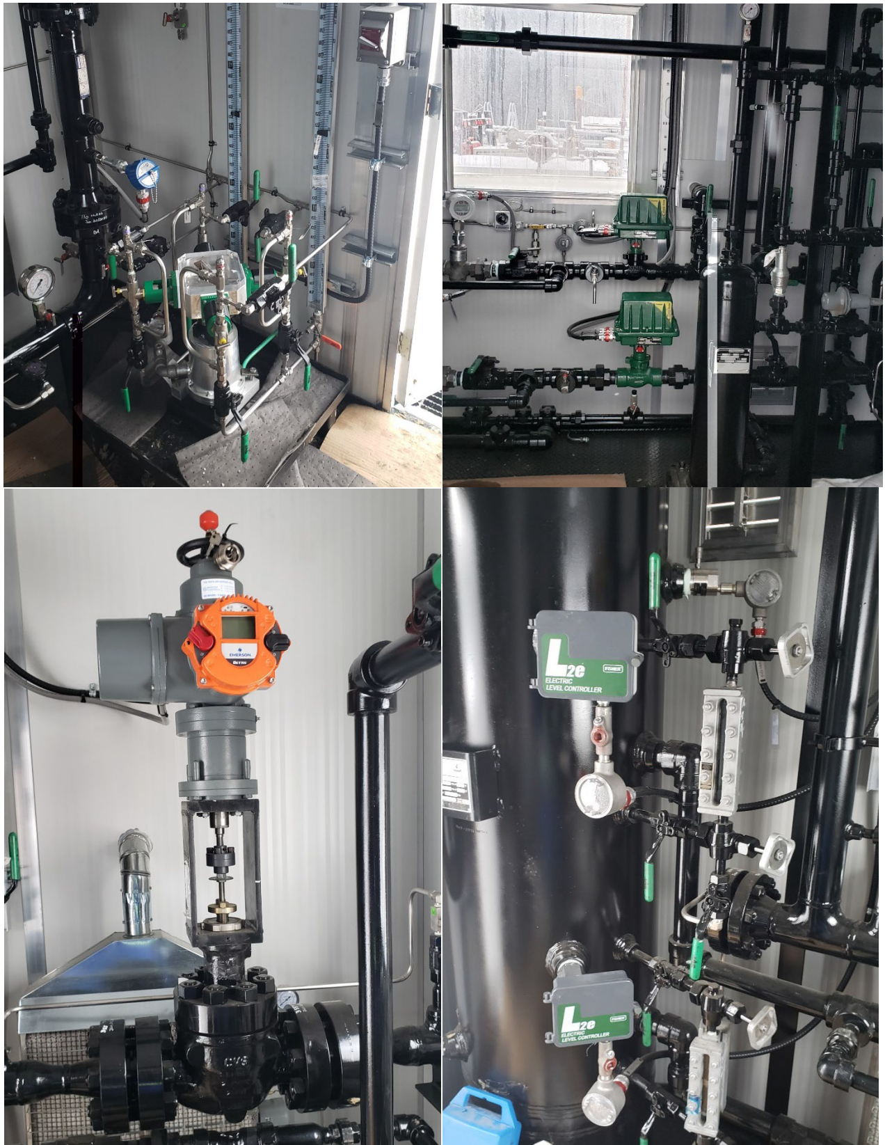
Figures 1-4: Electric Package A – [clockwise from top left] (1) LCO Crossfire electrical chemical injection pump, (2) Fisher D3e level control valves, (3) Fisher L2e level controllers, (4) Bettis RTS FL-05 inlet control valve actuator
