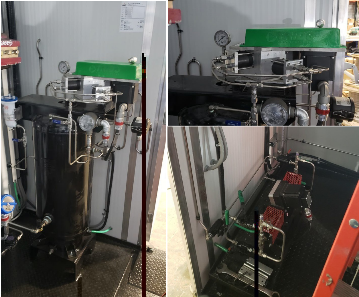
Figures 9-11: Instrument Air Package – [clockwise from top left] (9) Trido electric air compressor package, (10) Trido electric air compressor, (11) Trido electric chemical injection pump
