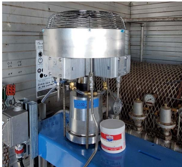
Figure 1: Installed CROSSFIRE air compressor
