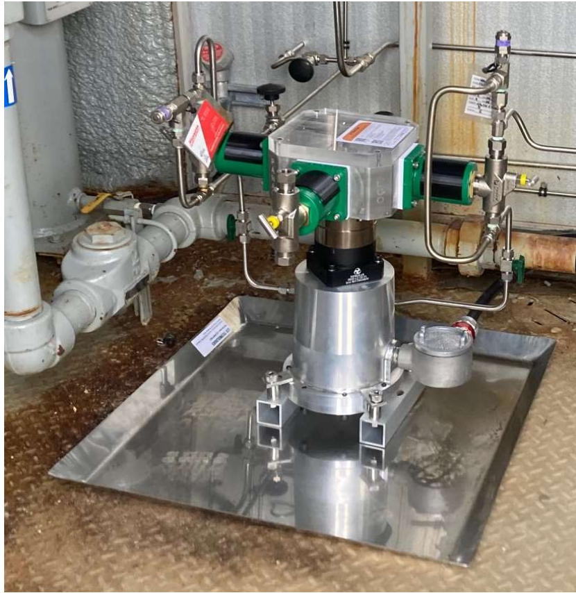
Figure 1: Installed CROSSFIRE chemical injection pump
