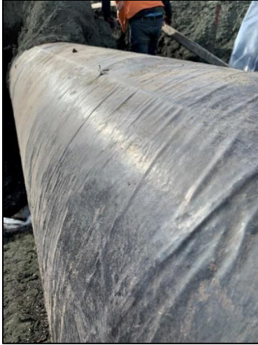
Figure 3-3: Minor tenting along pipe seam, MP 27.5276.
