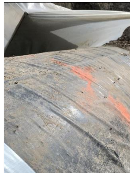
Figure 3-10: Tenting along pipe seam, MP 29.52
