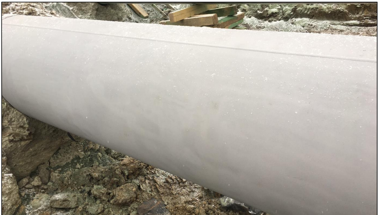
Figure 3-22: Pipe Surface at 3 O'clock Position
