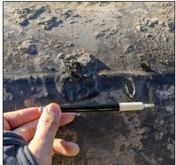
Figure 3-14: Disbonded coating at 1 o'clock position, MP 80.4655.
