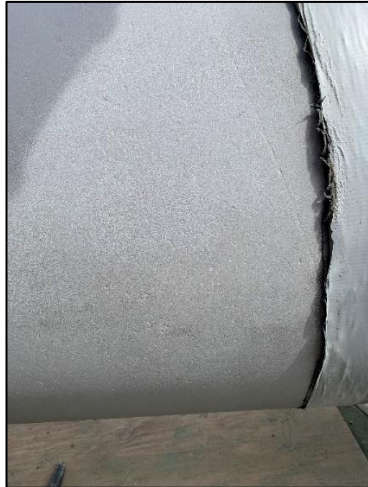
Figure 3-17: Pipe surface, 9 o'clock position, MP 29.52.
