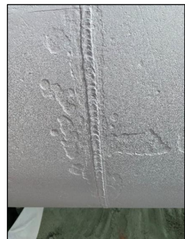
Figure 3-15: Wall loss near girth weld at 9 o'clock position, MP 27.5276
