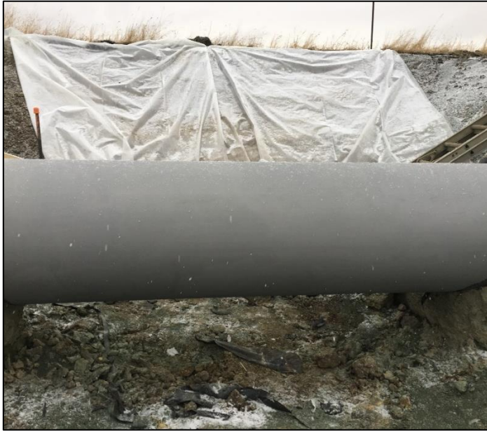
Figure 3-20: Pipe surface at 9 o'clock position, MP 80.4655.
