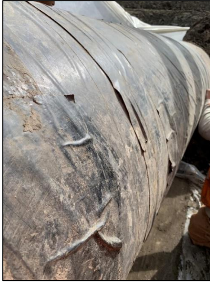
Figure 3-7: Moderate coating disbondment, MP 29.52
