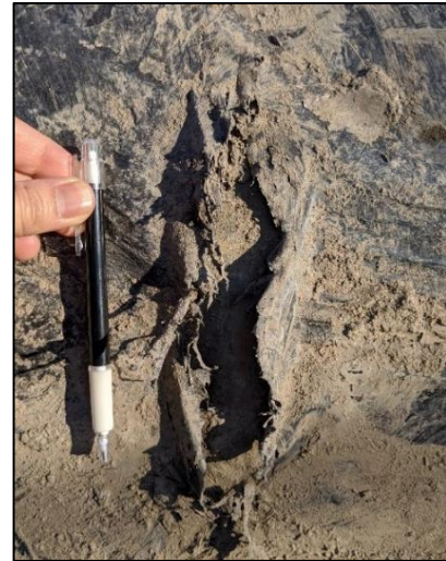
Figure 3-12: Coating damage at 9 o'clock position, MP 80.4655.
