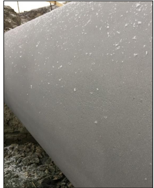
Figure 3-21: Minor pitting at 9 o'clock position, MP 80.4655.
