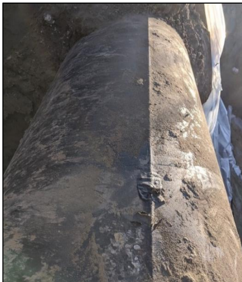
Figure 3-13: Tenting disbondment along pipe seam, MP 80.4655.
