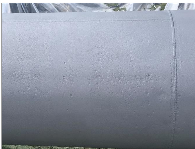
Figure 3-14: Clustered pitting corrosion and wall loss along girth weld, MP 27.5276
