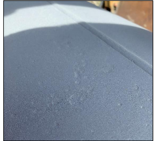
Figure 3-18: Corrosion features at 12 o'clock position, MP 29.52
