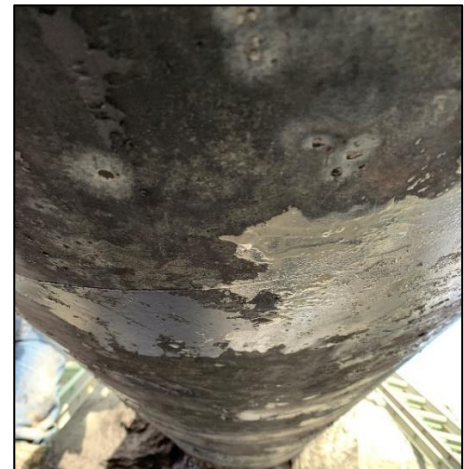
Figure 3-6: Moisture trapped on underside of pipe, MP 27.5276.
