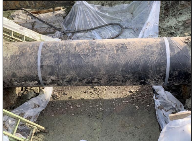
Figure 3-4: General circumferential wrinkling of coating, MP 27.5276.
