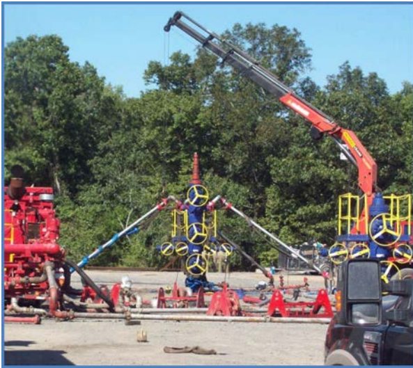
Figure 5: Wellhead Set Up for Hydraulic Fracturing Operation
