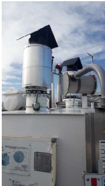
Figure 39 – Ferrier (15-16) 03-02-038-06W5 Condenser Vent
