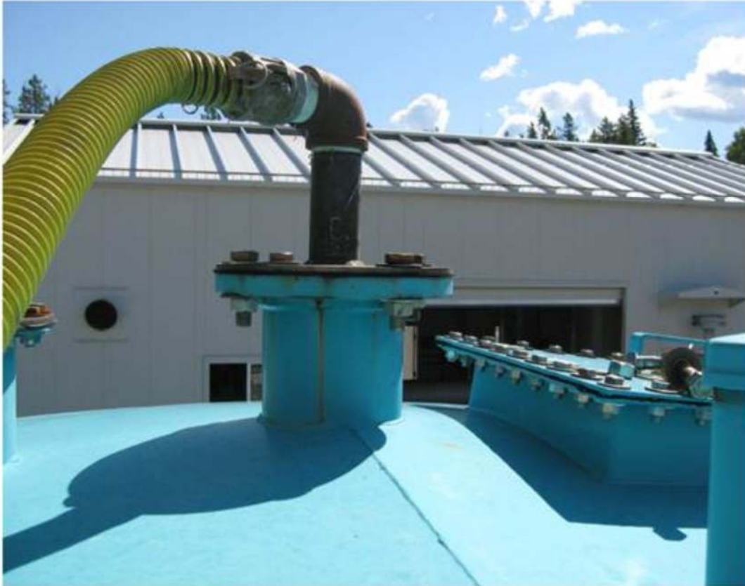
Figure 12 –TankSafe Overhead vapour collection using TCT Procedure (Source: Exova)
