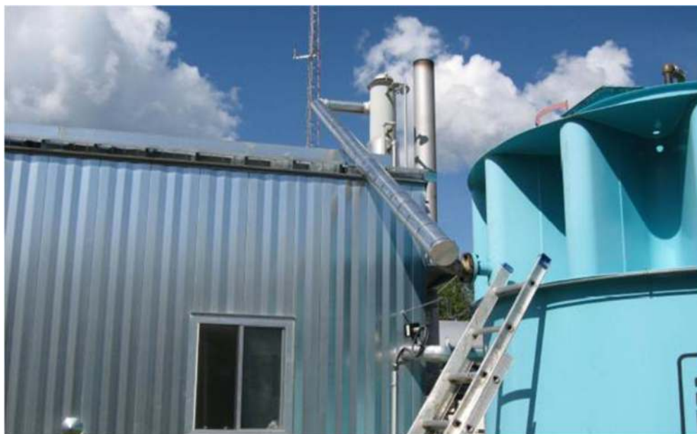
Figure 10 – Tie-in of Still Column Overhead to Tank Vent (Source: Exova)
