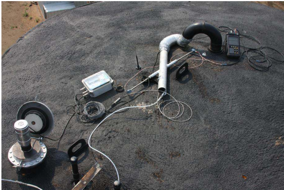
Figure 14 - Vent Emission Monitoring System (Source: Clearstone)
