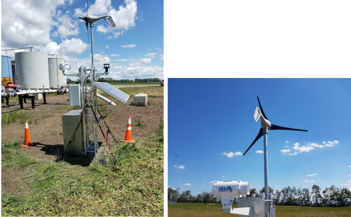
Figure 1 -Pictures of RMLD-REM installed at project test site. Left: Transmitter and receiver station with control box. Solar and Wind powered. Right: Transmitter and receiver are combined in one unit. Reflective target not shown.
