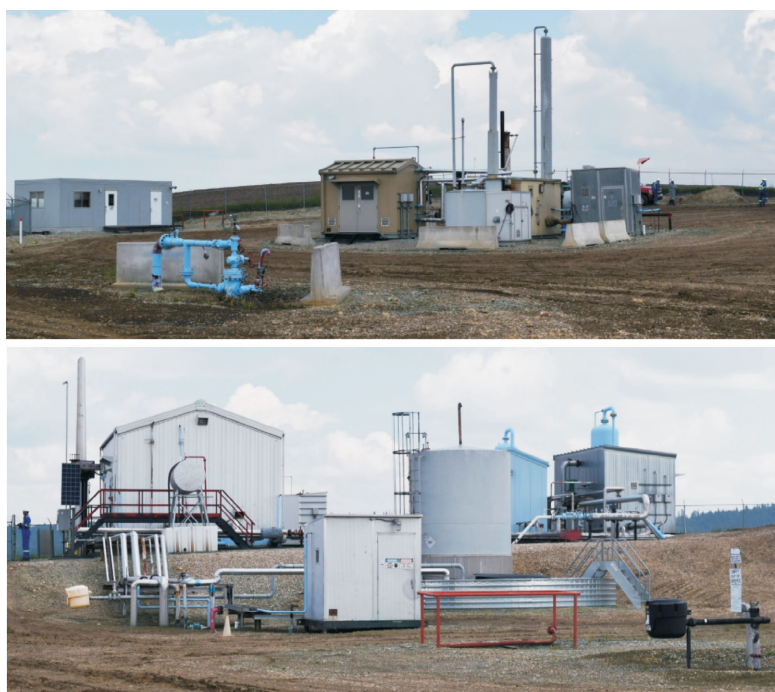
Figure 14. Facilities at Alberta Methane Field Challenge site 22.
