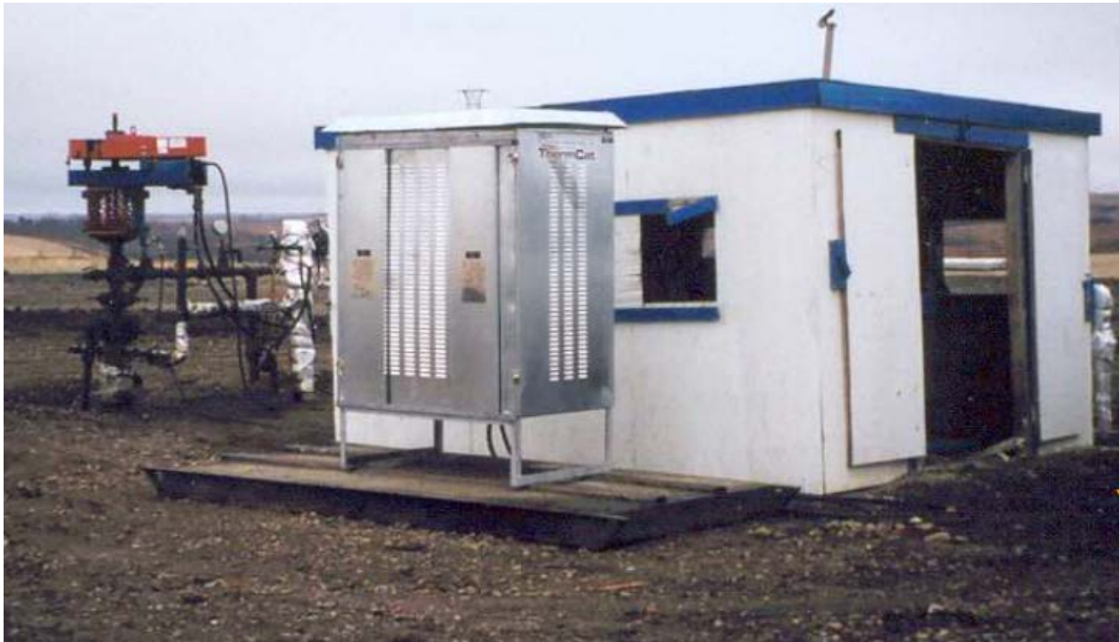
Figure 15: Field installation of a catalytic conversion unit (New Paradigm Engineering Ltd).
