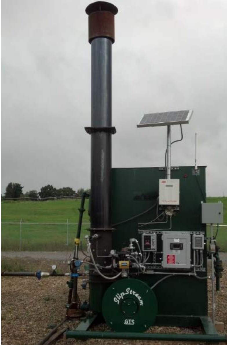
Figure 7: Installation of a SlipStream® GTS control system and auxiliary burner (Spartan Controls).
