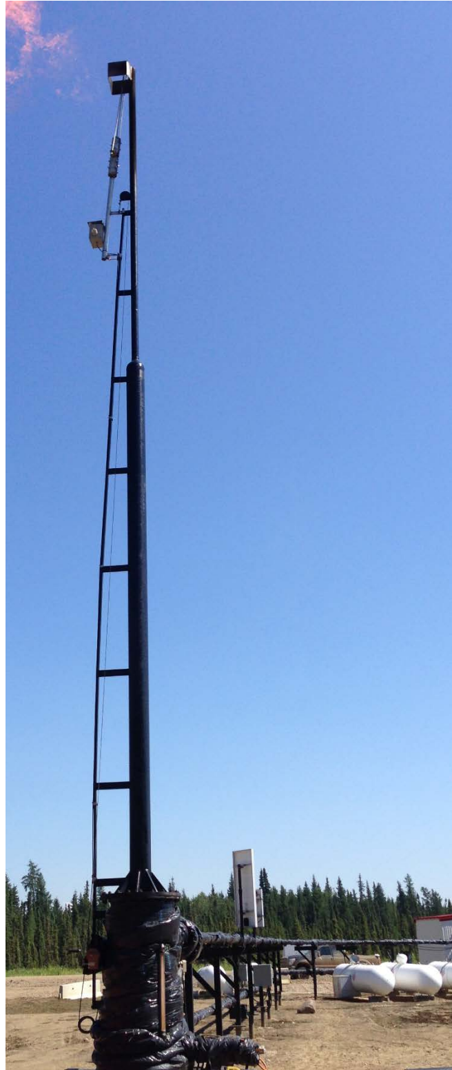
Figure 19: A shielded-flame flare stack with integral knock-out drum.
