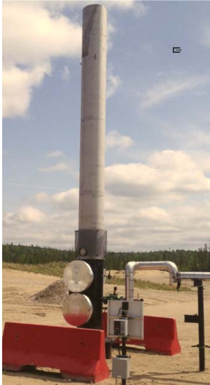
Figure 23: Field installation of a BGR 24 vapour combustor (Black Gold Rush Industries Ltd.)
