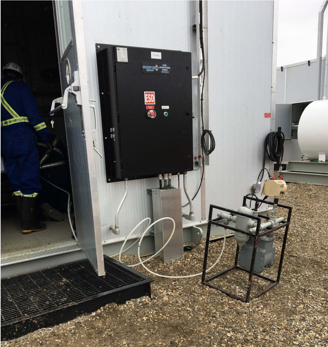
Figure 9: Calscan Hawk Meter Deployed at Site
