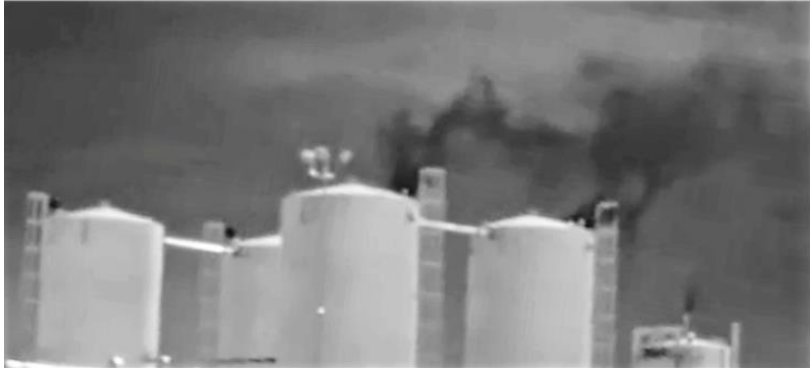
LSD 12-31 Storage Tanks FLIR Gas FindIR Image
