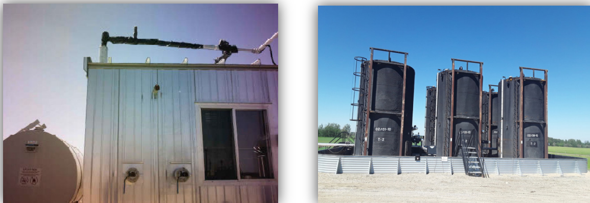
Figure 18. Well shack (left) and production tanks (right) at Site 8-8 with methane emissions.
