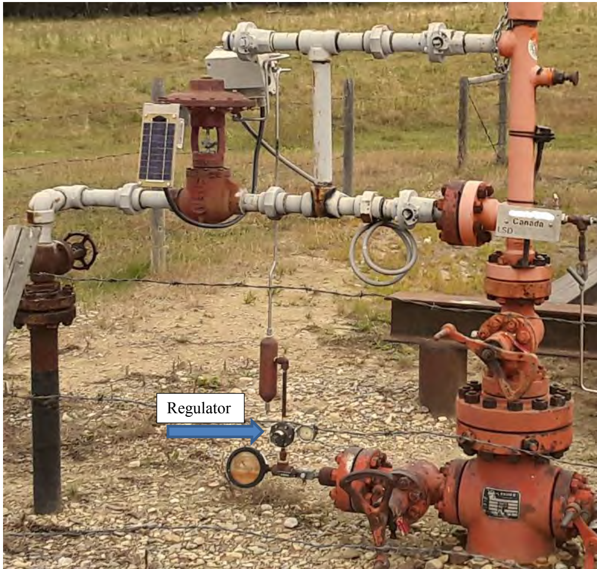
Figure 13: Example of a gas regulator installed on an oil wellhead.
