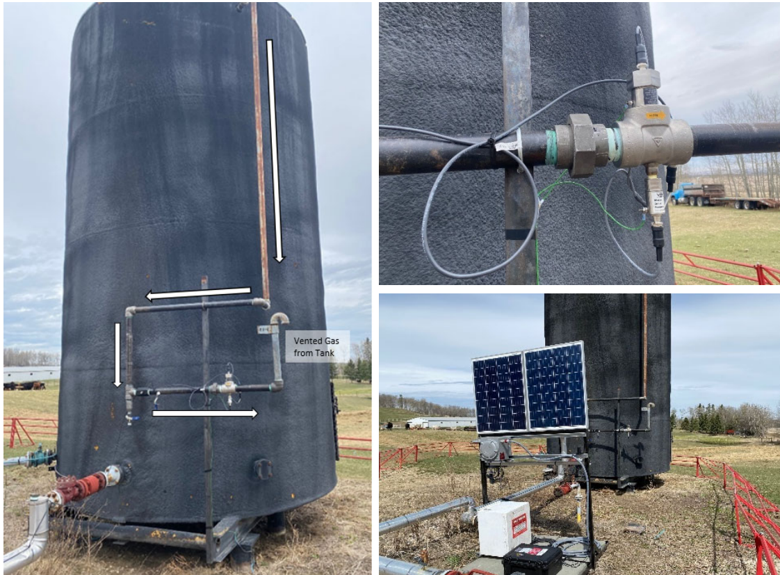
Figure 5: Ventsentinel® meter installed on 400-bbl tank with remote monitoring infrastructure to remotely data log the ongoing flow measurements and other measurement variables
