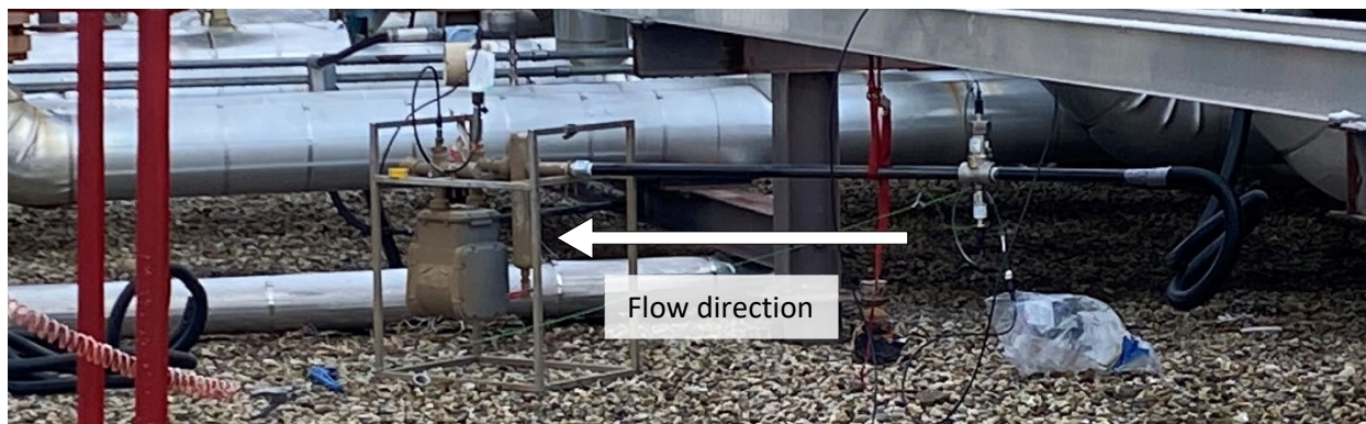
Figure 2: Flow Test Setup - Calscan Hawk 9000 and 1-inch Ventsentinel® installed at compressor station
