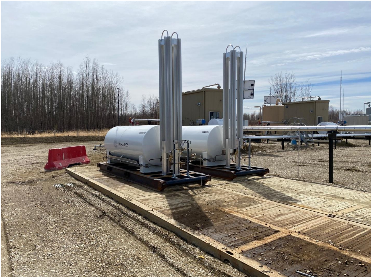
FIGURE 7: INSTALLED DEMONSTRATION UNITS
