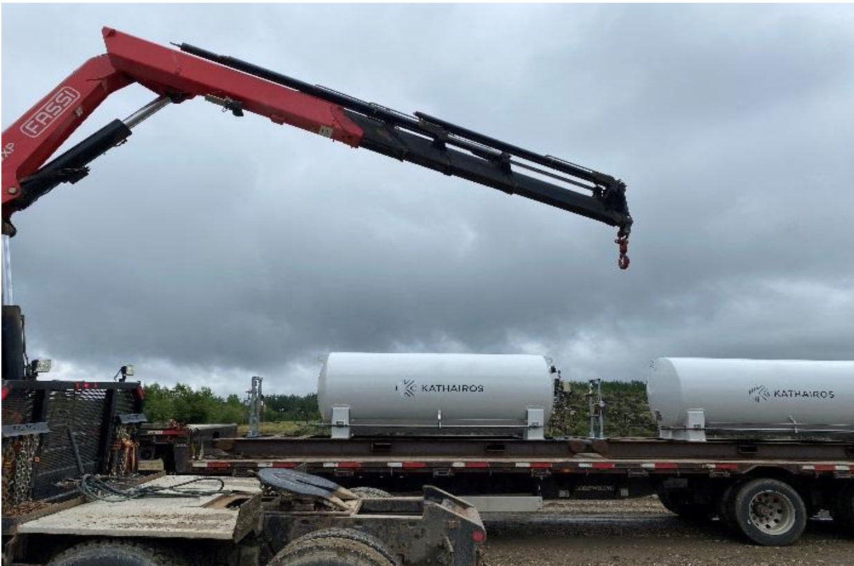
FIGURES 5 &6: INSTALLATION PHOTOS
