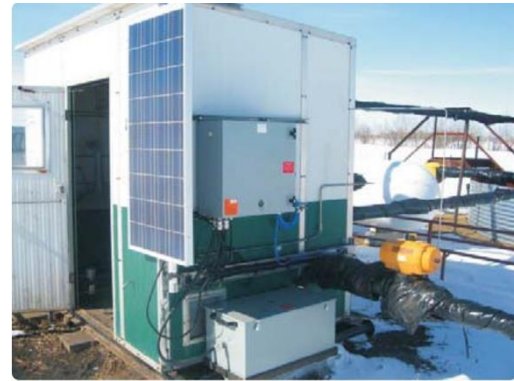
Retrofitted Separator with Bear Solar Electric Control System
