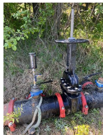
Leak-detection sensors evaluated under field conditions
